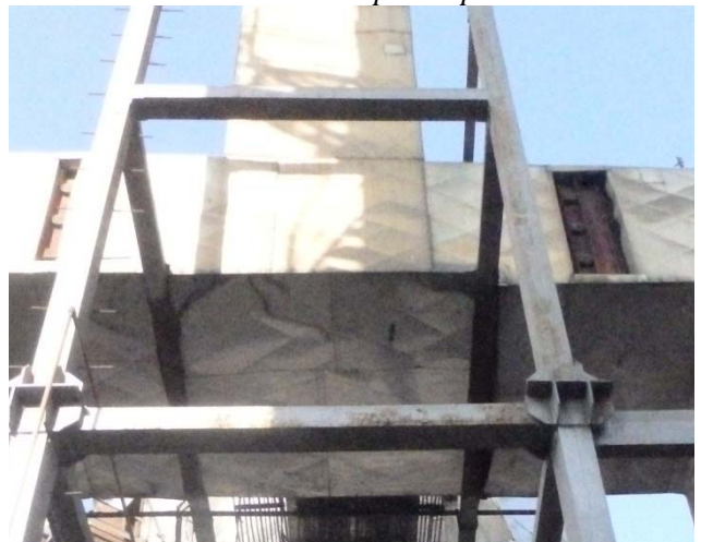
Photo 27: Uninsulated isolation dampers at ID fan inlet duct.
