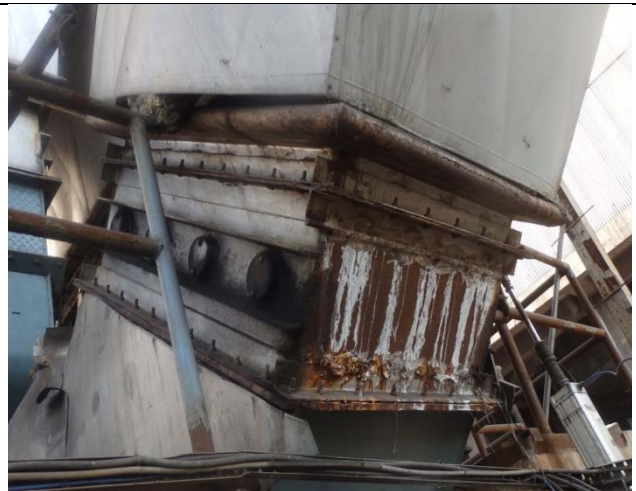
Photo 35: Flue gas condensation in uninsulated ducts, bellows and dampers. Removable pad insulation could be used.
