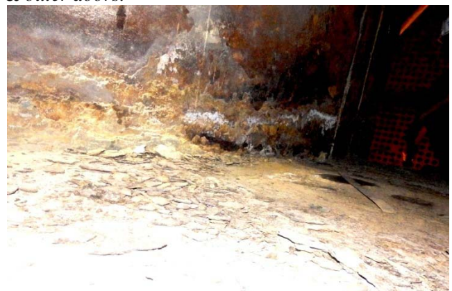
Photo 33: Corrosion due to uninsulated duct at fabric expansion bellow at ESP outlet.
