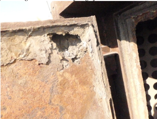
Photo 28: Air ingress in ESP inspection door caused corrosion.
