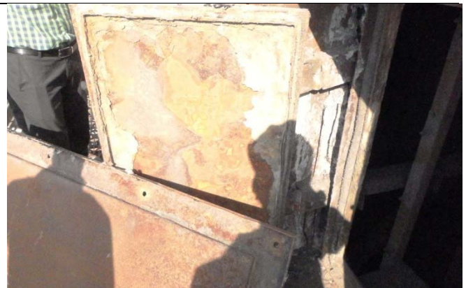
Photo 31: Flange leak in ESP double door system. Mineral wool mattress must be packed between inner & outer doors.
