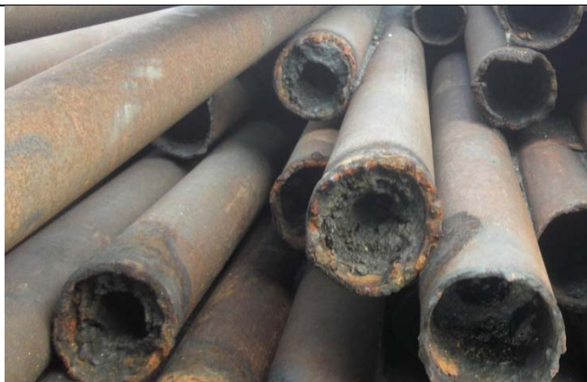
Photo 1- Plugging of airpreheater tubes. Unable to be removed.
