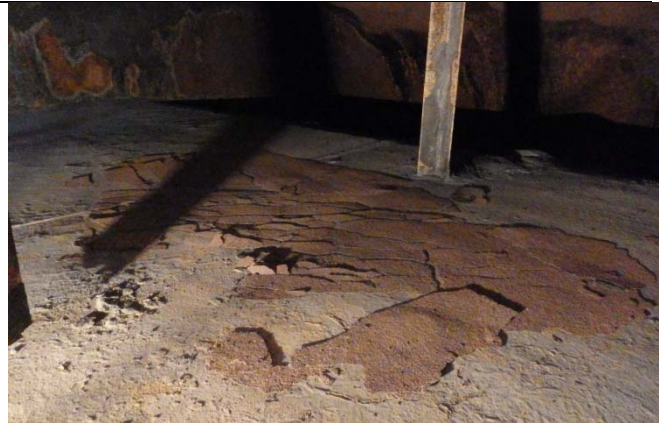
Photo 25: Corrosion APH top duct plate.
