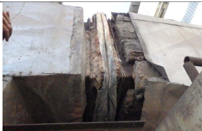
Photo 2: Flange leak, Fabric torn at NMEJ at boiler outlet.
