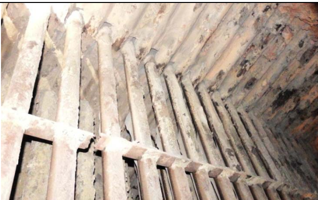
Photo 7- Air ingress marks are seen in SH area.
