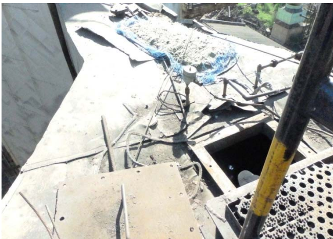
Photo 36- Improper inspection door at ESP inlet gas duct as source of water stagnation at top plate of APH - ESP duct. Double door system is needed here as well.
