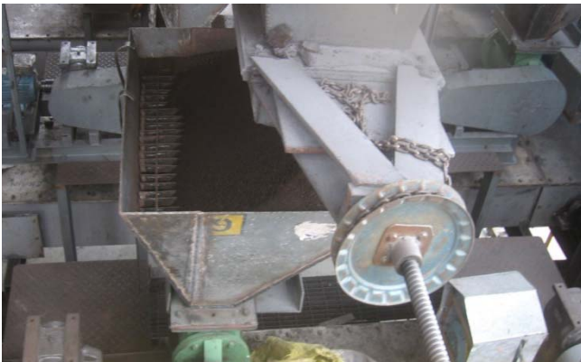
Photo 18: Static screen to arrest the lumps / foreign material going to feeder.
