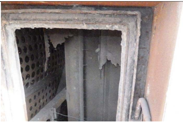
Photo 30- Corrosion of collecting electrodes in ESP due to localized condensation by air ingress from improperly sealed inspection doors.
