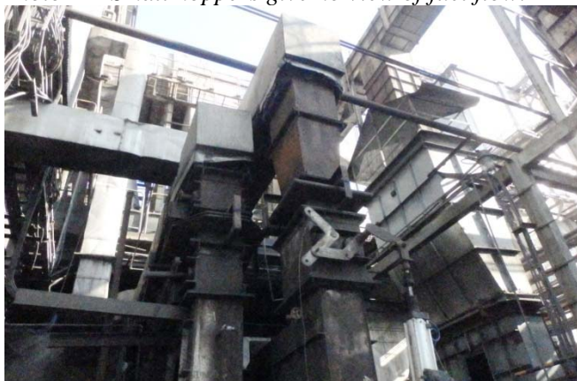
Photo 14: Multi flap dampers located immediate to PA fan outlet, affect fan performance.
