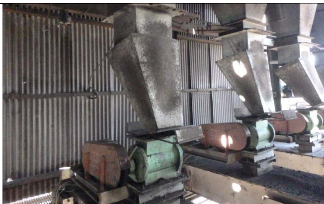
Photo 12- Small hoppers give no view of fuel flow.
