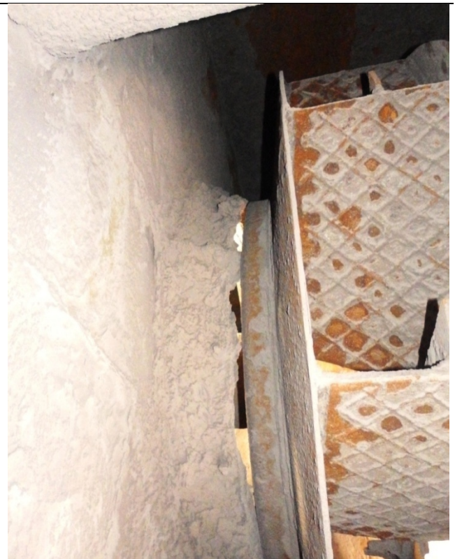
Photo 23: ID fan impeller eye to suction cone clearance / overlap not OK. Corrosion is the reason.
