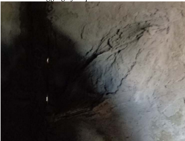
Photo 26: Air ingress at isolation damper flange joints. Light is seen at the flange joints.
