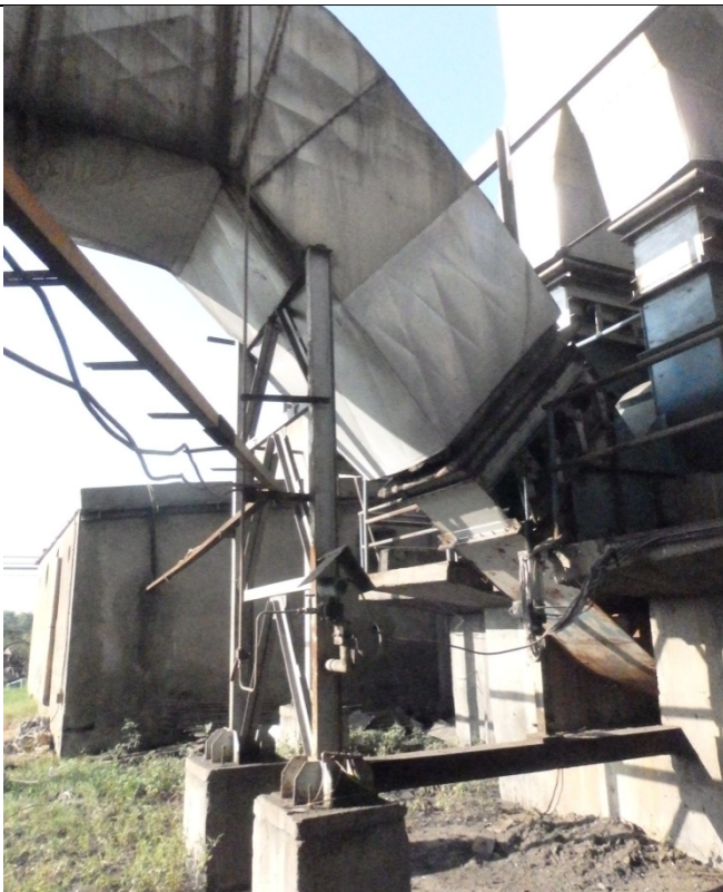
Photo 22- Draft transmitters wrongly installed at ID fan discharge.
