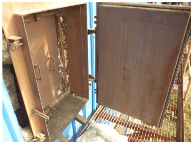
Photo 37- ESP double door systems also need proper sealing. Mineral wool mattress must be packed between the inner and outer doors.
