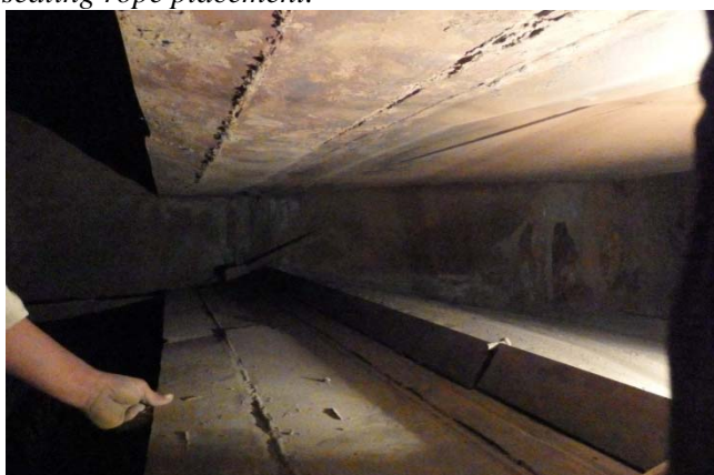
Photo 5: High velocity at Eco to APH duct is seen here. Below protection plate is eroded.
