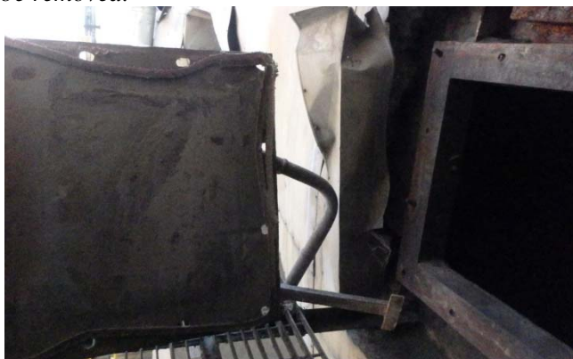
Photo 3: Air ingress at Inspection doors. Improper sealing rope placement.
