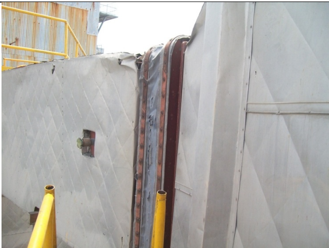
Photo 34- Fabric joint flanges are sources of flue gas condensation.
