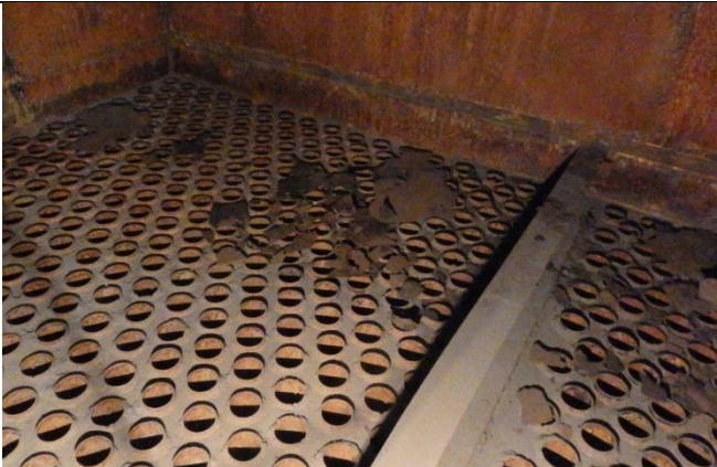
Photo 24- Plugging of airpreheater tubes.
