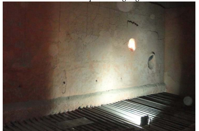
Photo 11: Better SA port arrangement. Less no and large pipes, on two side walls, provide proper penetration and combing effect.
