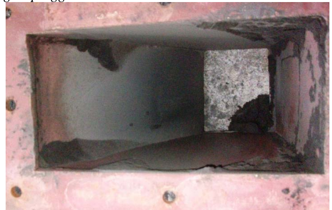
Photo 21: lumps formed at mixing nozzle chute due to +ve pressure at venturi.
