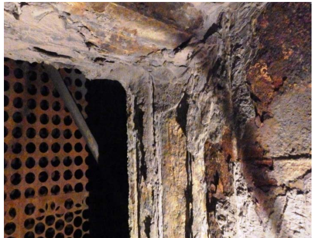
Photo 29: Air ingress in fabric joint flanges at ESP inlet.
