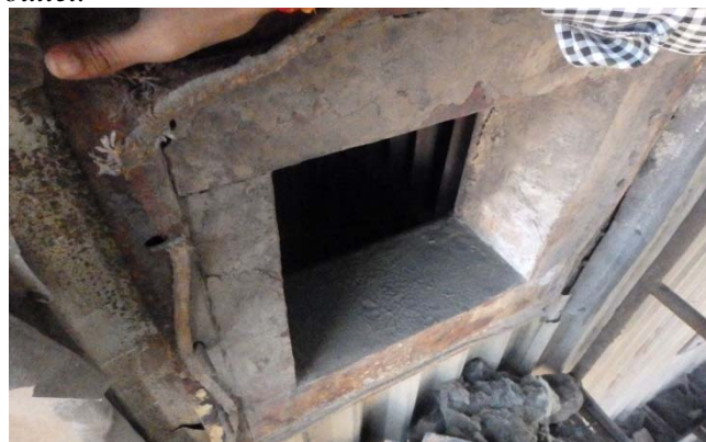
Photo 4: Air ingress in SH inspection door. Improper sealing rope placement.
